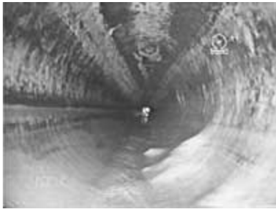
Figure 1 :: A lining showing small areas of inward folding.
