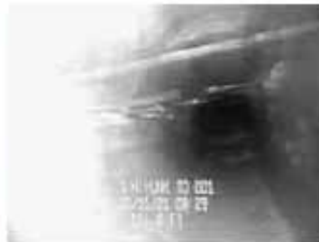
Figure 2 :: More extensive leak.
