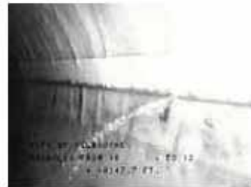
Figure 3 :: Severe leak with water jetting through seam.
