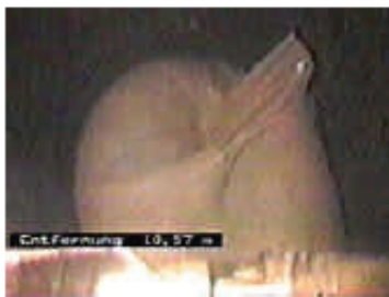
Figure 1 :: Example of stuck inversion with coated layer apparently trying to invert through split inner, note the cured section of seam.
