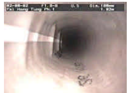
Figure 6 :: Example of air pockets behind the seam.
