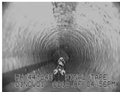
Figure 5 :: Increasingly severe undulating surface.
