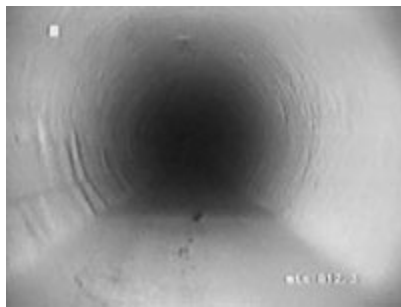
Figure 1 :: Slightly uneven finish at 7 o'clock pulling across a seam.
